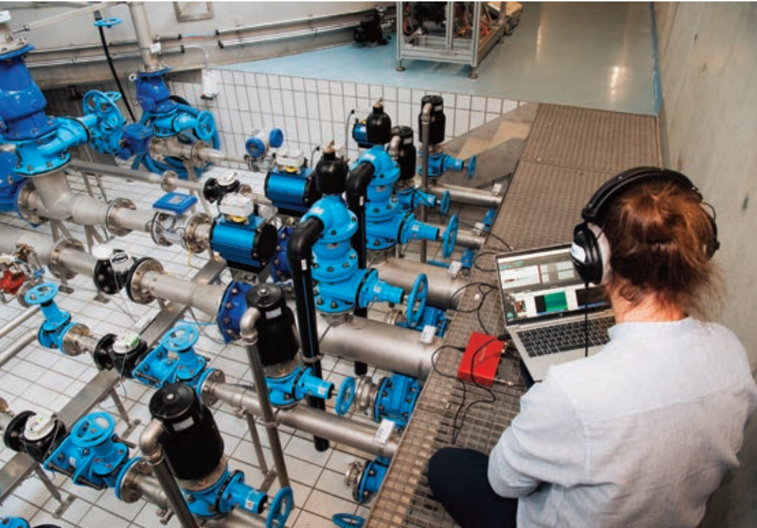
Valve field at the ZHB Weinleiten, which is monitored using body and air sound microphones and an infrared camera
